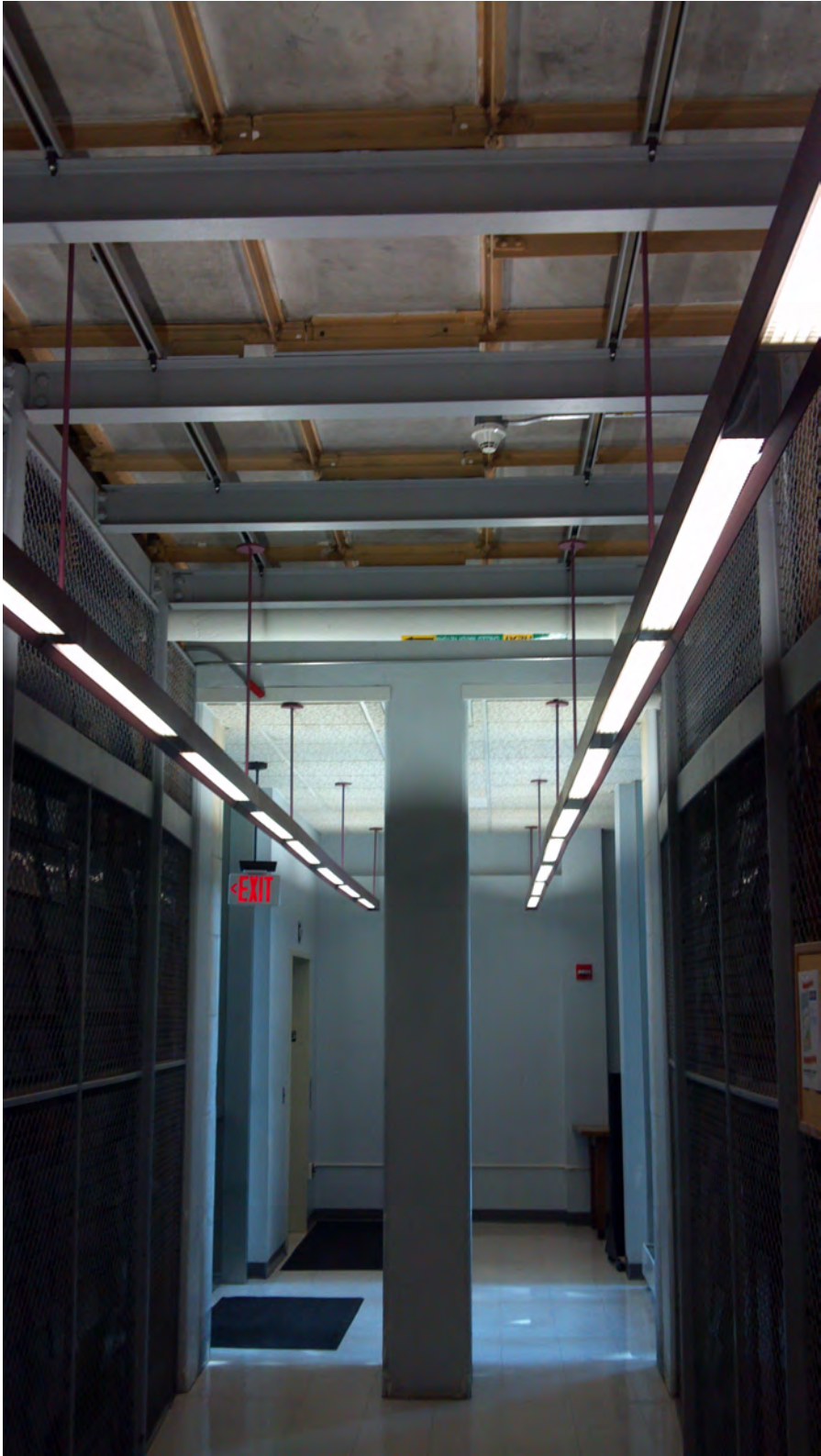
Hallway cut through the stacks on lower level (note underside of floor panels at top):
